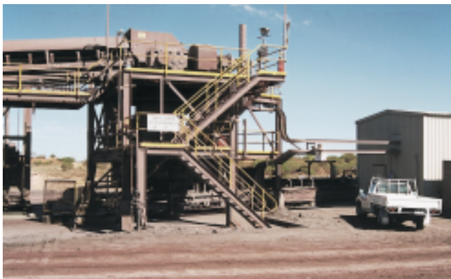
Conveyor plant drive unit
